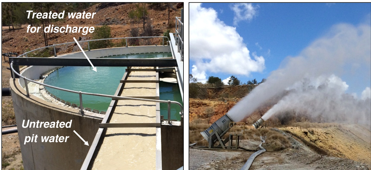
Figure 2: Operating water treatment plant and evaporators at the Mount Morgan Mine
